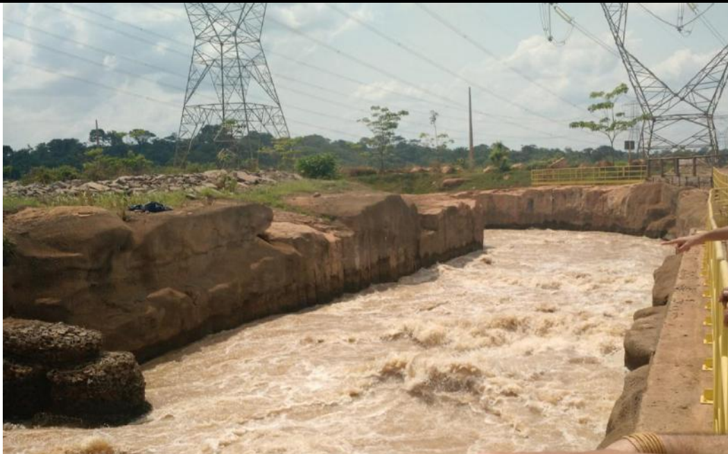
Picture 2. Picture of one of the channels showing the FTS in the operating period.
